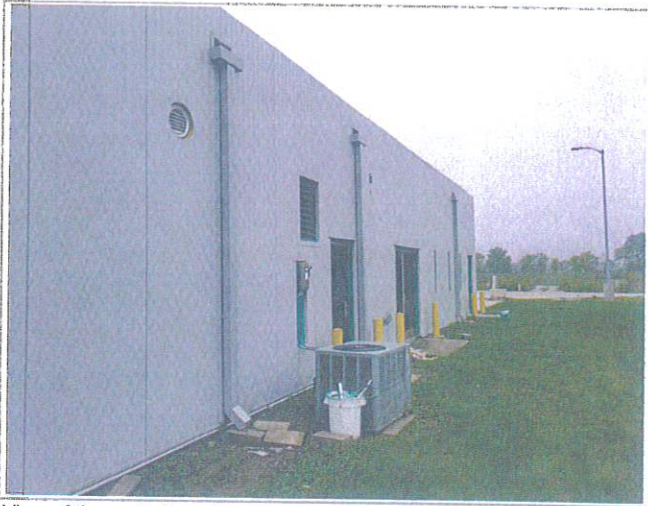
View of the north face shows roof membrane has been pulled back as work continues around roof edges; New downspouts have been fabricated and installed
