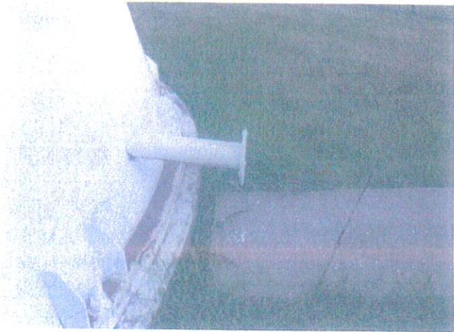
Overflow Pipe Termination
