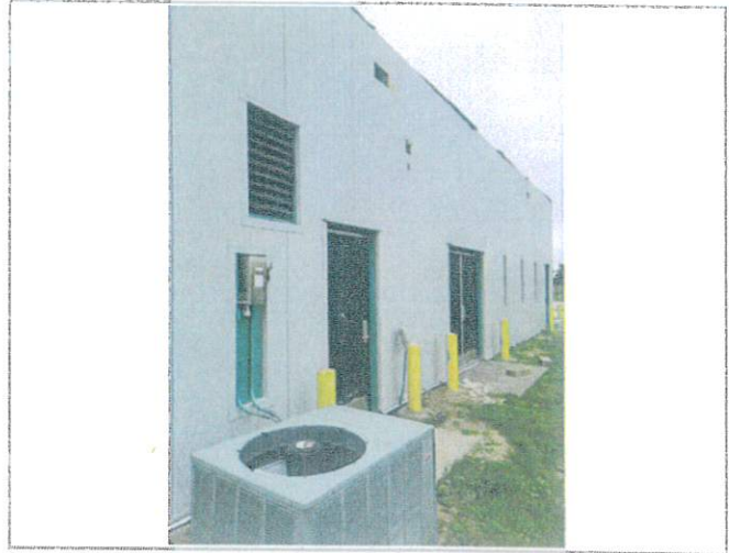
Overview of the north face shows trims have been applied around doors, windows, louver and electrical box; it was discussed the exposed green vapor barrier will be painted over to match building
