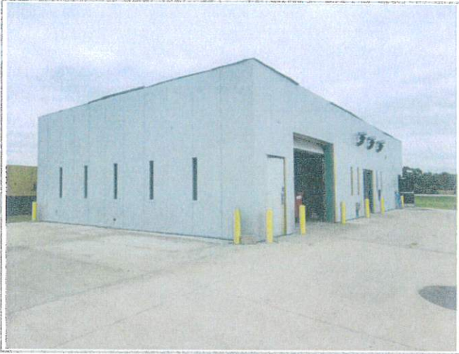
Overview from SW corner of site, shows trims progressing around the building - windows are trimmed out on the west windows; south windows need trims; coping materials are being fabricated;
