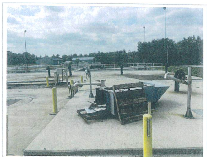
Demolished RTU remains onsite
