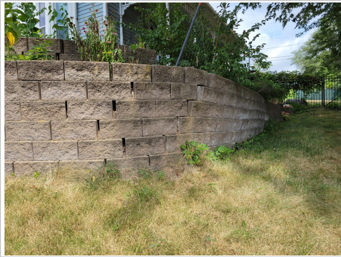
Pictures of existing retaining wall prior to construction and in poor conditions with separation in blocks and forward tilt of wall face.
