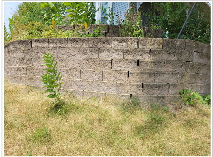
Additional pictures of existing wall in which you can see separation of block on both lower and upper walls, as well as tilt in fence behind lower wall.
