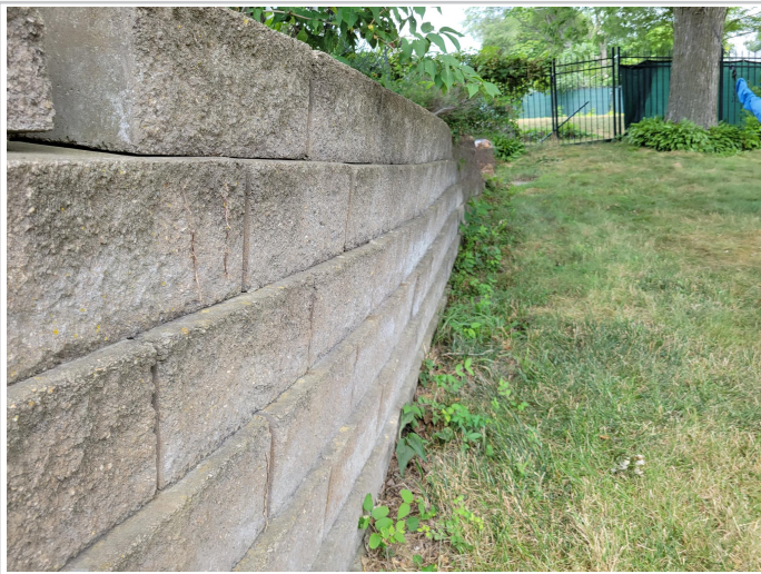
Zoomed in picture of existing retaining wall, depicting tilt forward of wall face.
