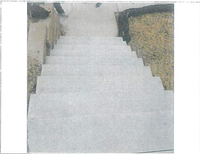
The new stairs were questioned in terms of rise and run being with code. Each stair was measured and has been verified that with design standards and construction code.
