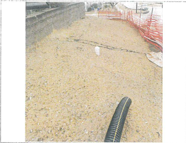
Sanitary sewer cleanout is exposed and will remain exposed so that it can be accessed and maintained as needed. This is typical and standard.
