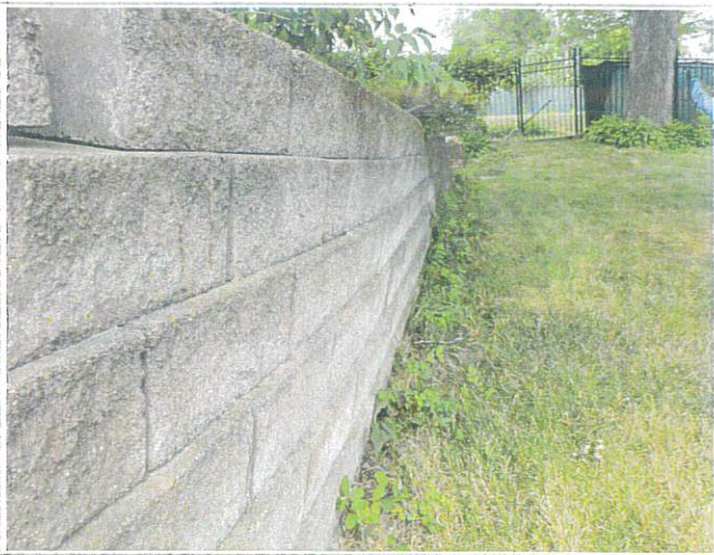
Zoomed in picture of existing retaining wall, depicting tilt forward of wall face.
