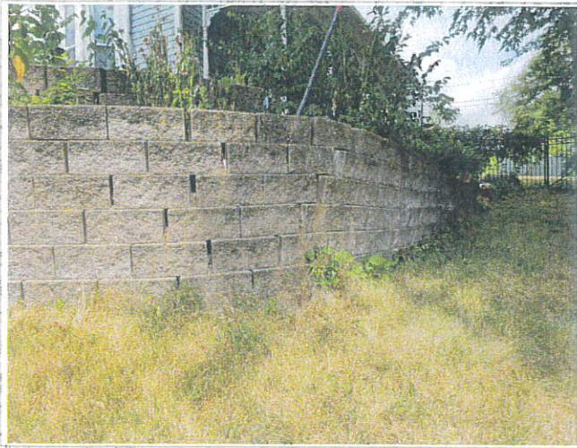
Pictures of existing retaining wall prior to construction and in poor conditions with separation in blocks and forward tilt of wall face.
