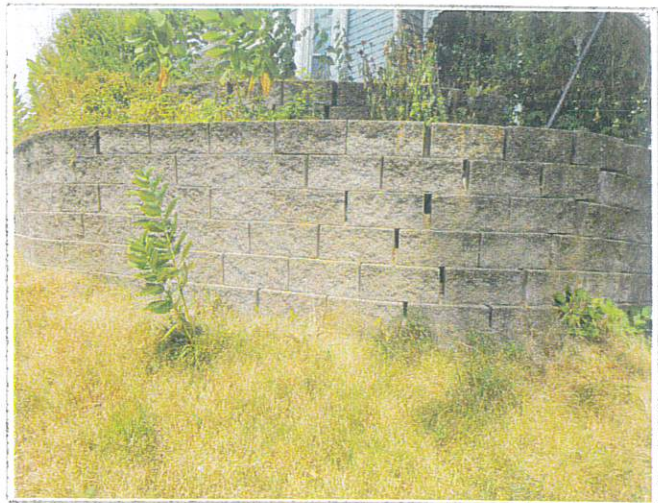
Additional pictures of existing wall in which you can see separation of block on both lower and upper walls, as well as tilt in fence behind lower wall.
