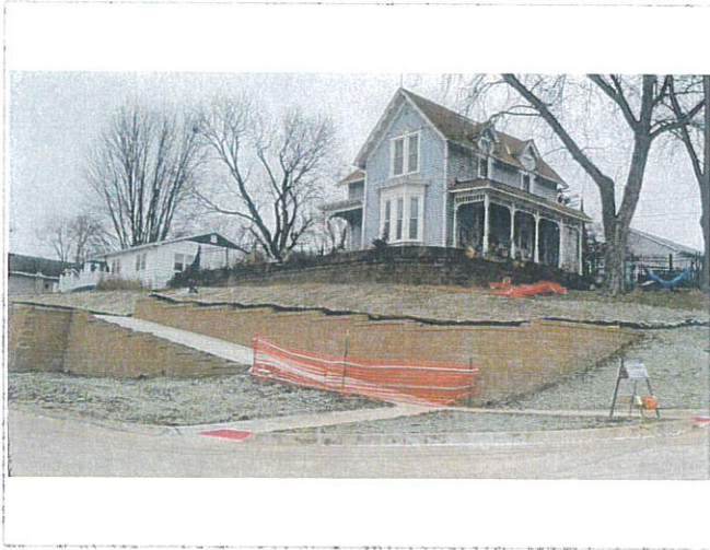
Requesting that some type of safety rail or fence be placed on top of the retaining wall within the private property.
