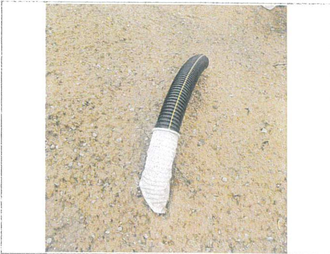
Subdrain cleanout and termination point. This tile will be cut down to grade and a cap placed at surface so not sticking up above ground.
