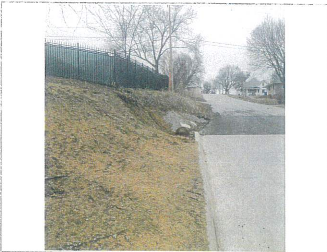
Final grading was questioned along the west side of Greene Street. It was noted by Axiom that grading and seeding is temporary due to winter weather. Additional grading and restoration is to be completed.
