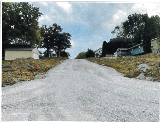
PCI has cored out and graded with road stone - looking east up Third Street from Washington intersection
