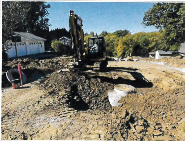
Carter & Associates backfilling new sanitary manhole 30 located just west of Glasgow and Third Street
