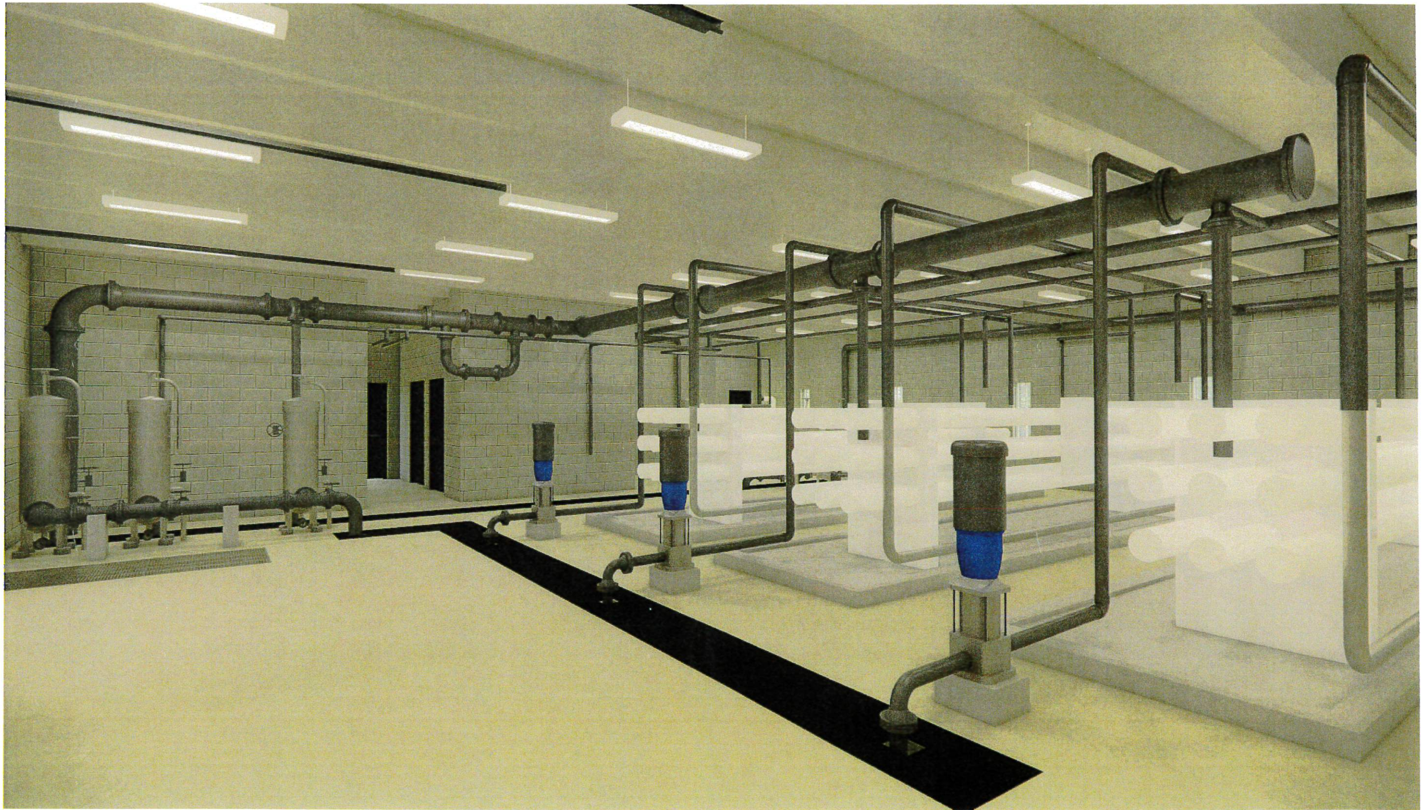
R.O. Feed Piping Riverside WTP Pipe Improvements
