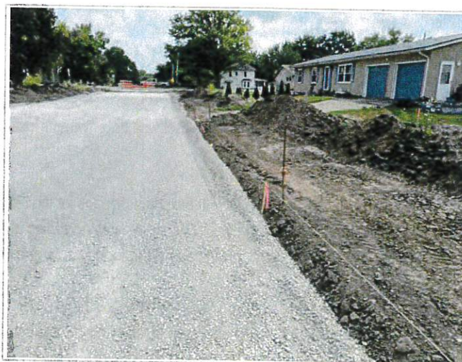
Streb has string-lines set throughout the rest of Phase 1 as they prep for upcoming paving
