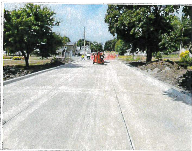
Concrete has been poured, cut and sealed from 2nd & Ella around to 2nd & Rose Streets
