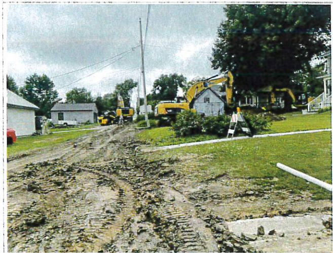
Crews re-working the sanitary sewer issues located in the alley off Rose Street
