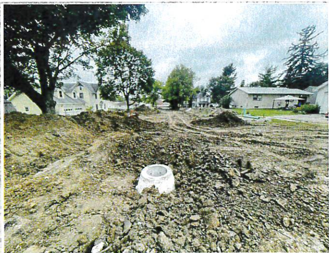
New sanitary manhole located at the north end of Rose and 3rd Street (near alley)
