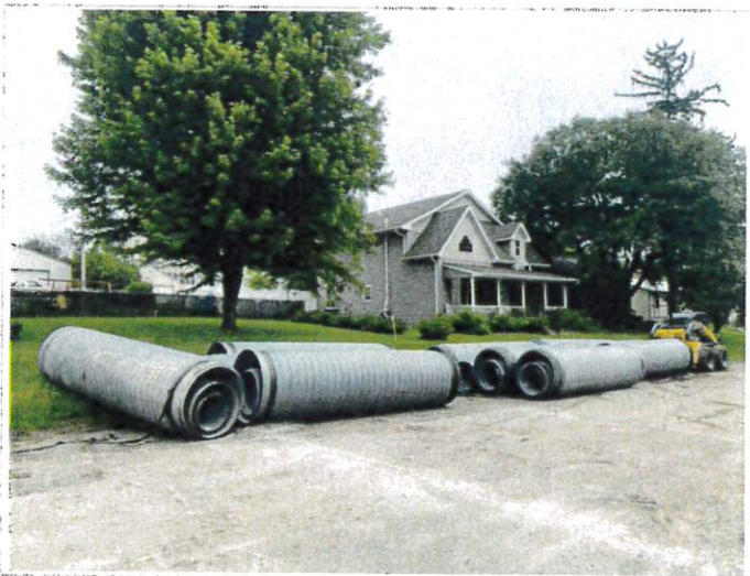
Materials starting to arrive and being staged at corner of 3rd Street and Ella
