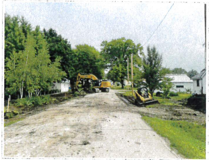
PCI working way north up Rose toward 3rd Street demolishing driveways and clearing out ROWs
