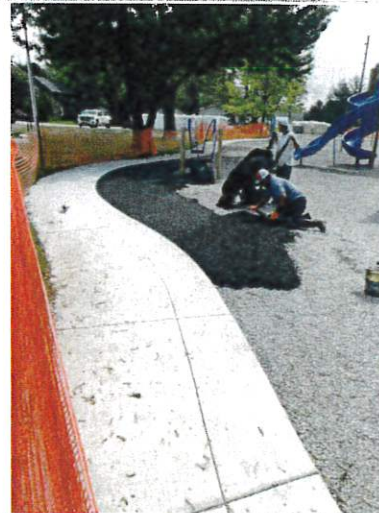
Playground surface base installation has started, top layer will follow after base has cured
