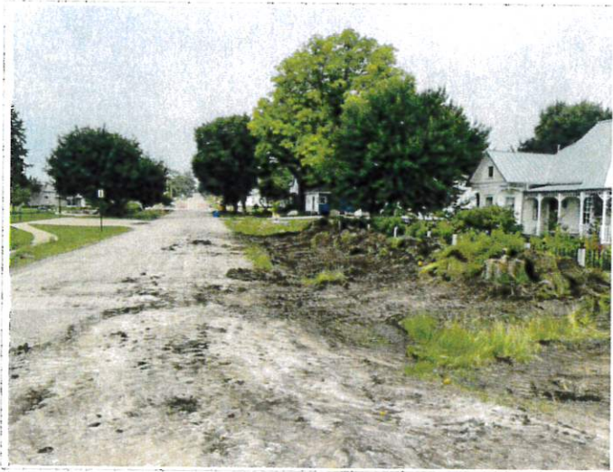
Looking west down 2nd Street from corner of Rose, PCI has started clearing out ROW for upcoming Utility work
