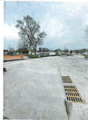
Overview of the west side of S Hickory along the park - shows parking and sidewalk has been poured and finished along the east side of the park since last reporting
