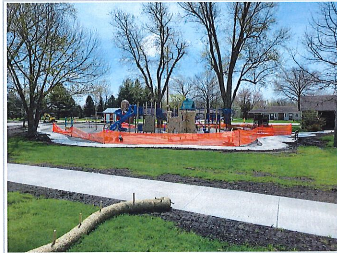
Looking south at the park, shows playground area being protected with construction fencing
