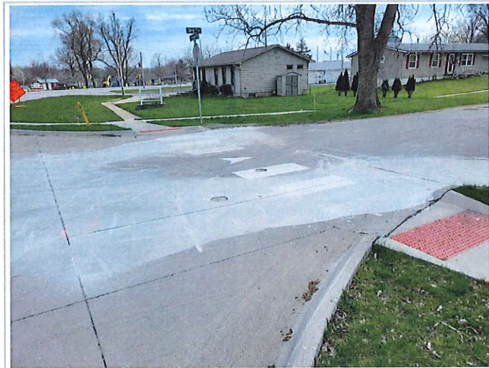
View of HWY 22 & Third Street, concrete cuts have been made at multiple points along Third Street to prep for removals
