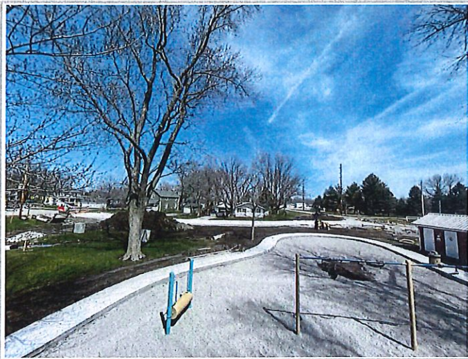
Center of park looking East over park sidewalk and Hickory. Subdrain installed throughout playground area. Park surface has been graded and prepped for the playground surface application
