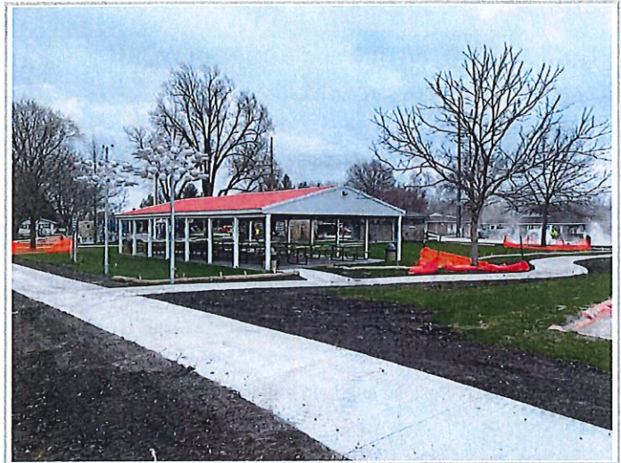
NW corner of site looking over completed sidewalk along 1st Street and West side of project.
