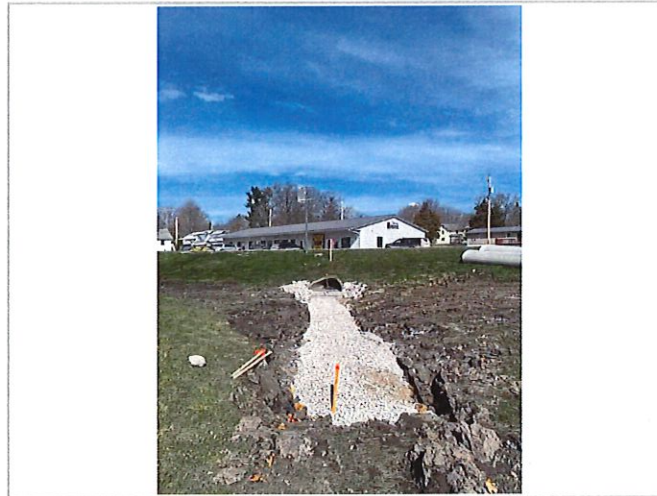
Location of where new storm line will be to take water from existing flared end section to proposed rain garden location.
