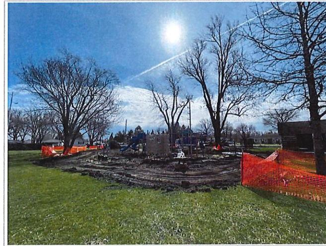
North of project site looking towards park. All sand removed by AAC and ready for subdrain installation by Maxwell.
