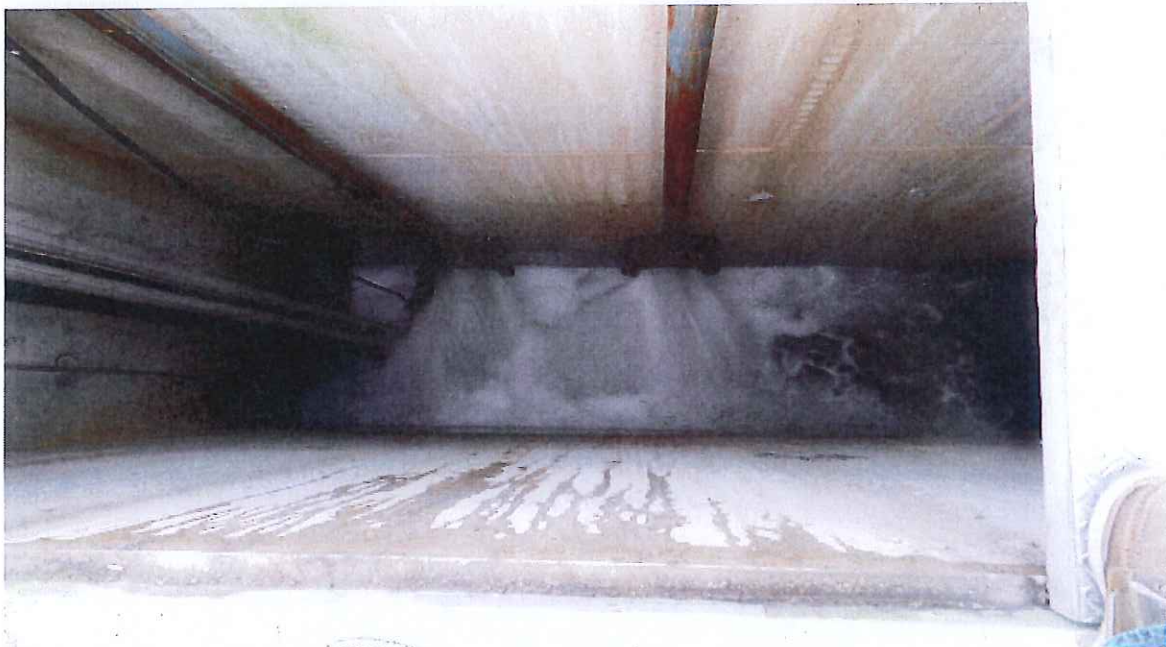
SBR 1 West Decanter Clear, East Decanter Clear After 30 seconds
