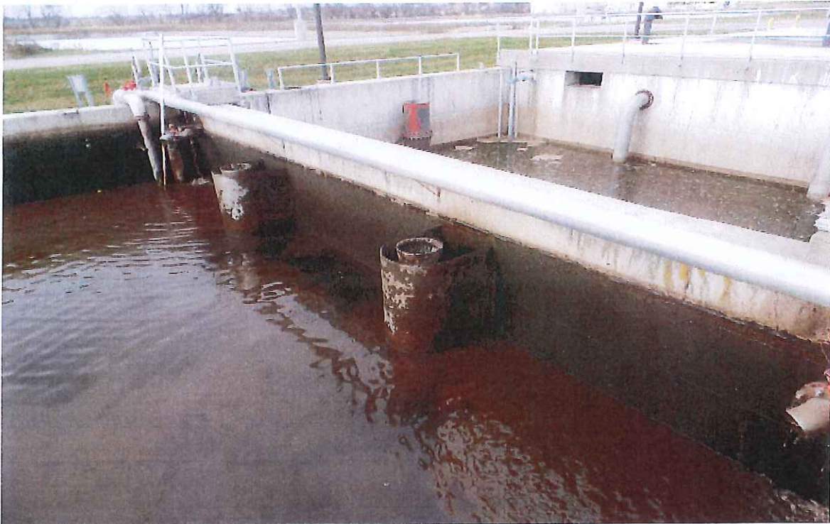
SBR 1 During Fill
